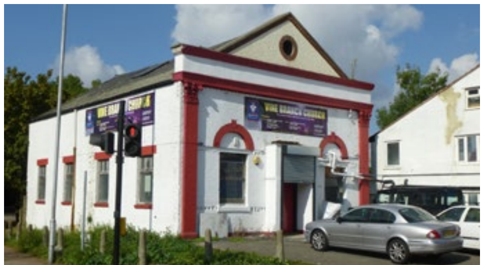
The Chapel is an attractive building but is in need of repair
