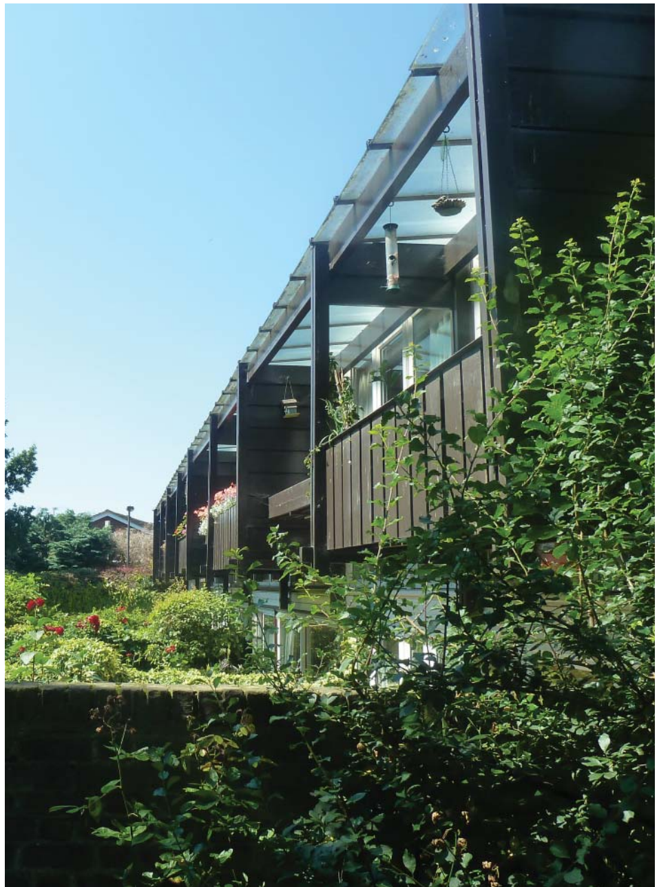
Well maintained southern elevation of a terrace of houses in St Bernards with important architectural features of balconies and timber panelling
