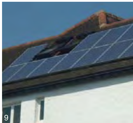
Solar panels visible from Ryecroft Road
