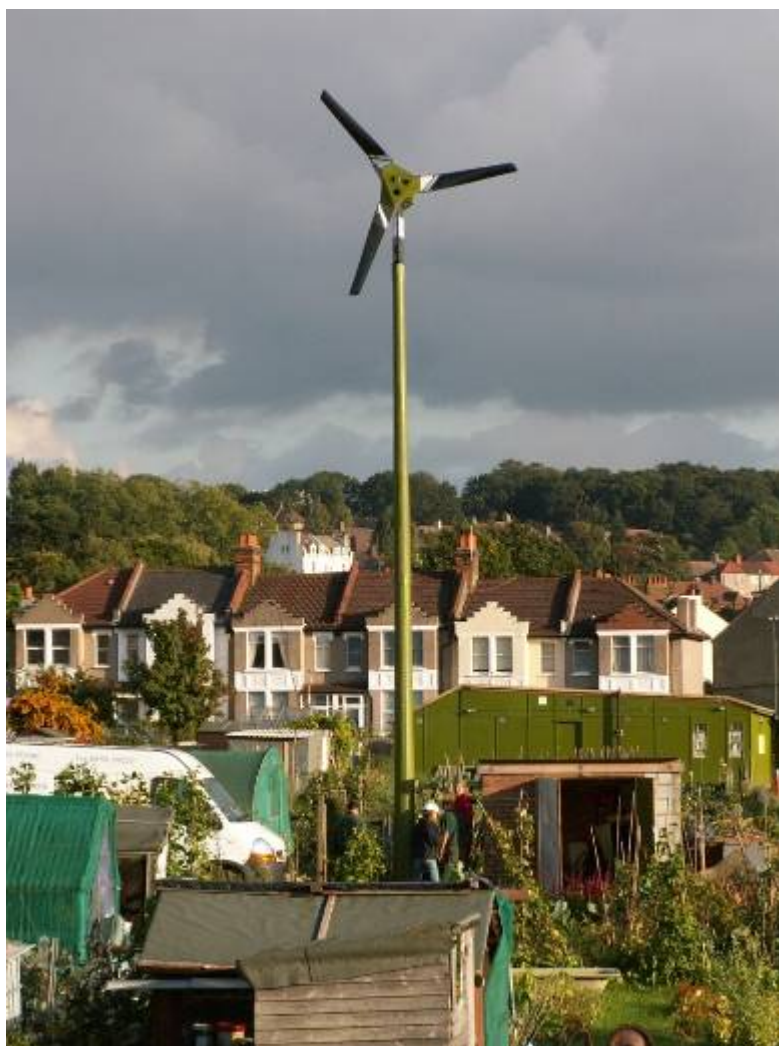
Figure 4: A 2.5 kW Proven wind turbine installed at Spa Hill Allotments
