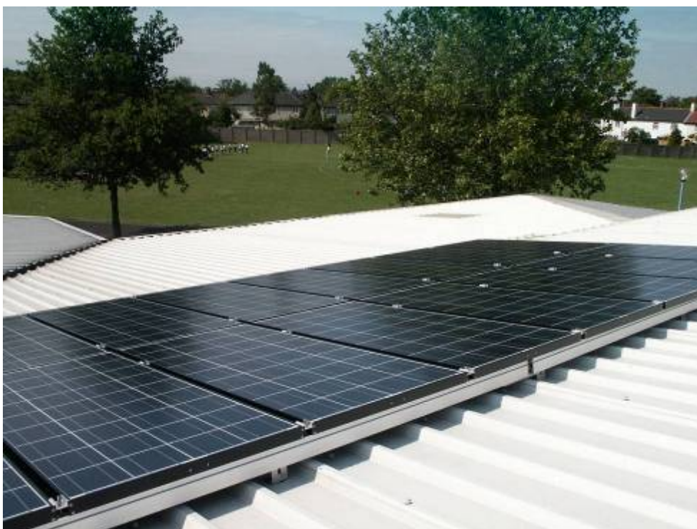
Figure 5: PV panels installed at Virgo Fidelis School
