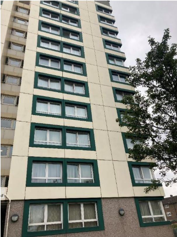
Fig 5 Southern elevation 2-56A showing render finish to ground floor to over-cladding and aluminium panels used for remainder of block
