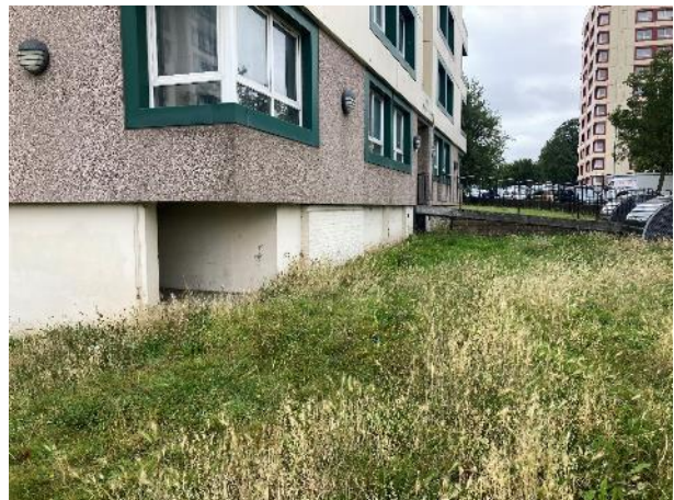
Fig 8 Low level south-eastern elevation 2-56A Showing render finish to ground floor to concrete and brick substructure
