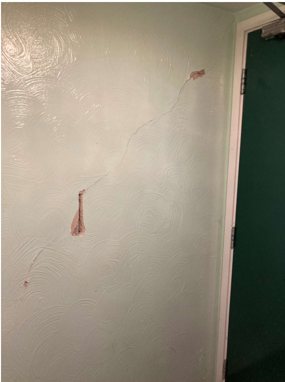
Fig 4 Diagonal crack in wall propagated through impact from door handle
