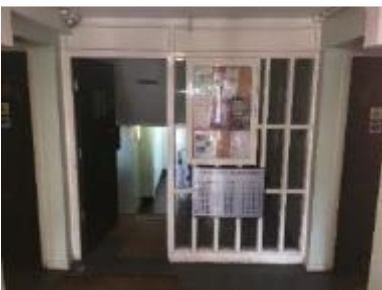
Figure 32 Fire door sticking open.
