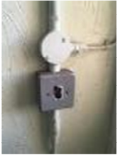
Figure 14 Damaged AOV test switch.
