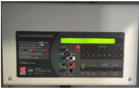
Figure 2 Fire alarm panel.
