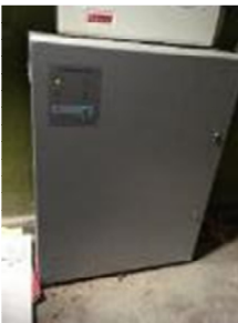
Figure 11 AOV control panel supply.
