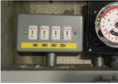
Figure 24 Multi gang emergency lighting test switch.
