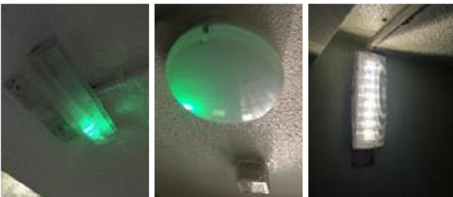
Figure 20 Typical emergency lighting.
