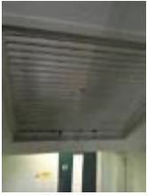
Figure 13 Primary stairwell AOV.
