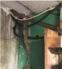
Figure 31 Disconnected earth bar.
