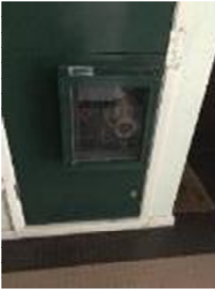
Figure 18 Dry riser outlet with no sign.
