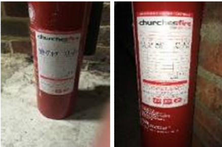
Figure 19 Extinguisher out of test.
