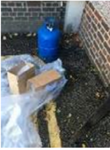
Figure 30 Rubbish stored outside the primary stair final exit.
