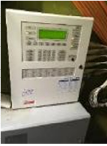
Figure 9 AOV control panel.
