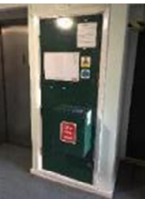
Figure 17 Dry riser inlet on ground floor.
