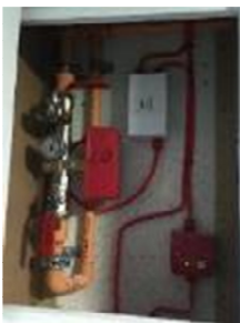
Figure 6 Sprinkler fire alarm interface.
