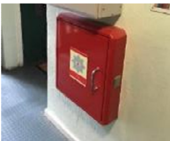
Figure 8 Fireman's information box.
